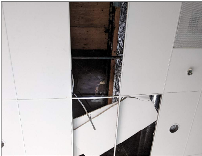
Figure 14 Damaged plywood area at
