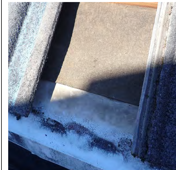
Typical anti-ponding metal properly lapped with underlayment at gutter edge of tile roofs.
