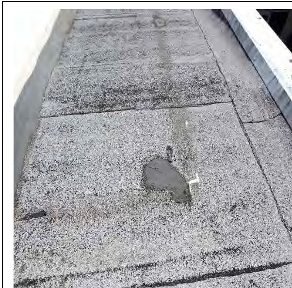
2.1A Roof sheathing is decayed. Note, previously patched holes. Location: Clubhouse
