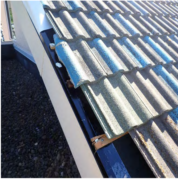
2.14A Tile is missing at rake edge of roof. Location: Bldg. 2
