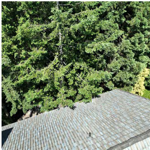
2.3 Tree extends over edge of roof. Vegetation should be trimmed back a minimum 2' from edge of roof.
