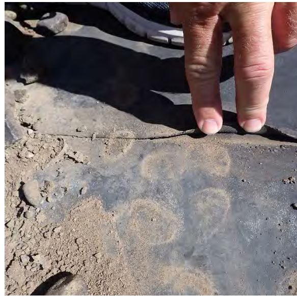
2.9A Seam at EPDM roof is lifting. All lifting or open seams should be repaired. Location: Bldgs. 1, 3, 4
