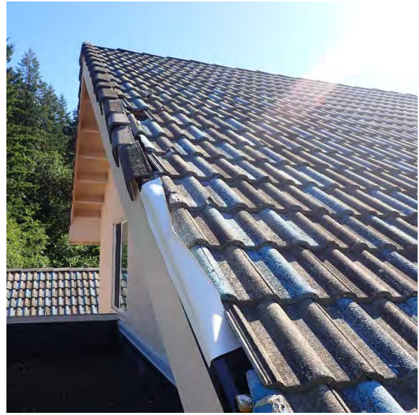
2.14B Additional view of missing tile at rake edge of roof.
