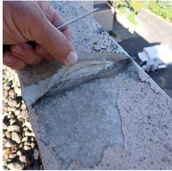
2.17 Sealant at coping metal joint is failing, and joint is lifting. Location: Bldg. 1
