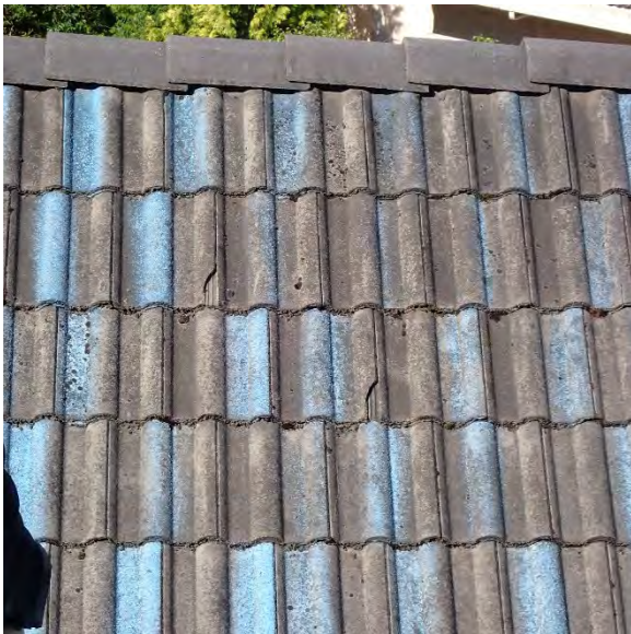
2.13A Lower corners of tiles are cracked and missing. Any tile with a crack over 3" should be replaced. Location: Systemic throughout property
