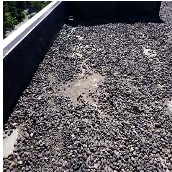
2.6 Gravel at EPDM roof is spread too thin, allowing the roof to be more exposed to UV and increasing the chance of the roof blow-off in these areas. Location: Bldg. 4
