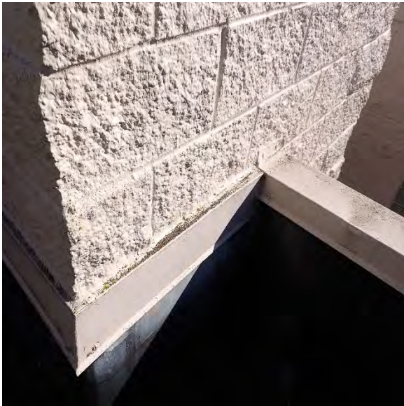
2.18A Surface mounted reglet and coping metal are sealant dependent at CMU wall and should be regularly maintained to ensure they remain sealed. Location: Systemic throughout property
