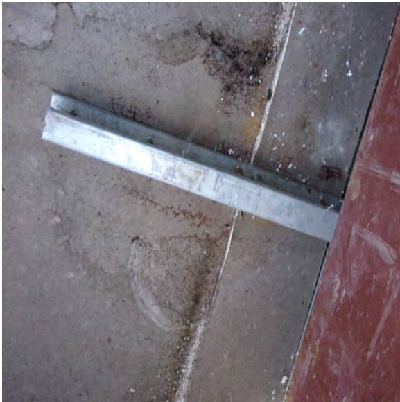
2.22C Water staining present on underside of roof hatch due to water intrusion at damaged handle.
