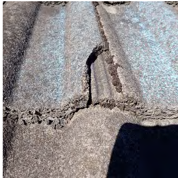
2.13B Closer view of damaged lower corner of tile.
