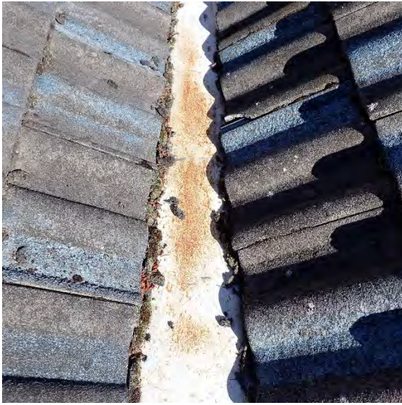
2.11 Low slope metal valley roof between tiles is corroded. Location: Bldg. 1
