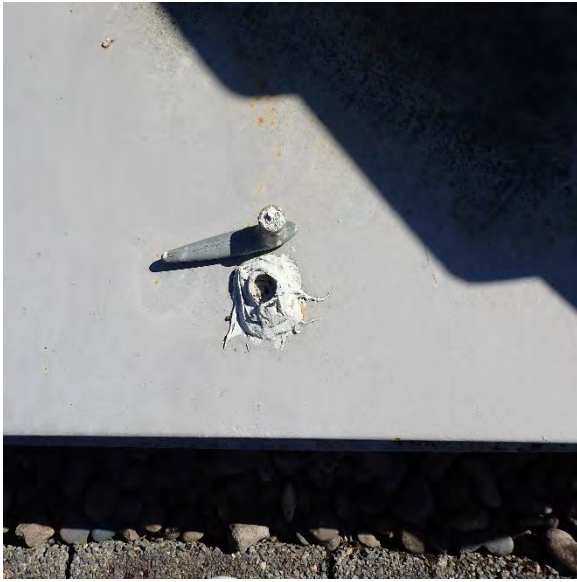
2.22A Handle at roof hatch is damaged and corroded, allowing possible water ingress. Location: Bldgs. 2 & 5
