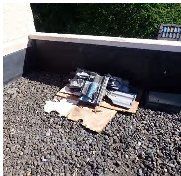
2.7B Additional example of debris from previous repairs present at EPDM roof.
