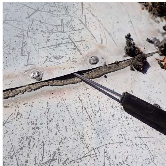
2.10 Open seam present at low slope metal valley roofs between tile roofs. All lifting or open seams should be repaired. Location: Bldg. 1
