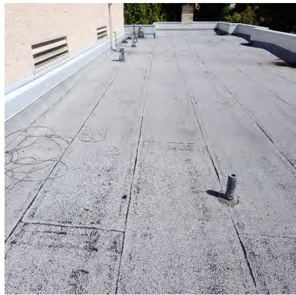
2.2 Granule loss is occurring on modified cap sheet sooner than typical. Further review is required to determine cause of premature granule loss.
