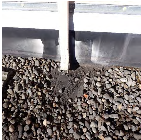
2.4 Splash blocks are missing at base of downspouts on EPDM roofs.
