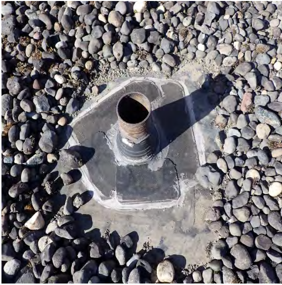
2.16B Additional example of previously repaired pipe flashing.
