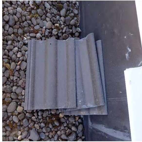
2.12 Extra tiles are being stored on roof. Tiles should be removed and stored in safe location. Location: Systemic throughout property
