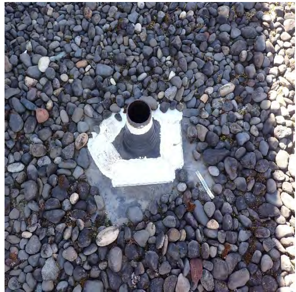
2.16A Pipe flashings on EPDM roofs have been previously repaired. Repairs to penetrations should be continued as needed until the roofs are replaced. Location: Systemic throughout property
