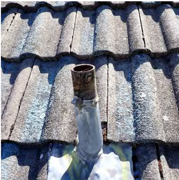
2.15 Lead cap at for pipe flashing is missing, allowing possible water ingress. Location: Bldg. 5
