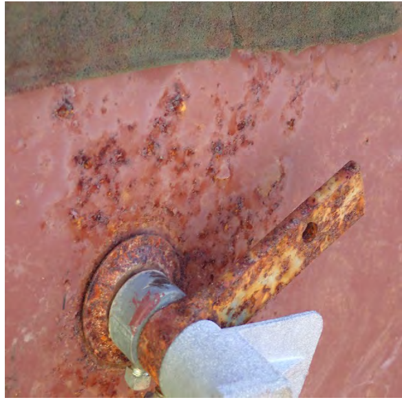
2.22B Additional example of damaged and corroded roof hatch handle.
