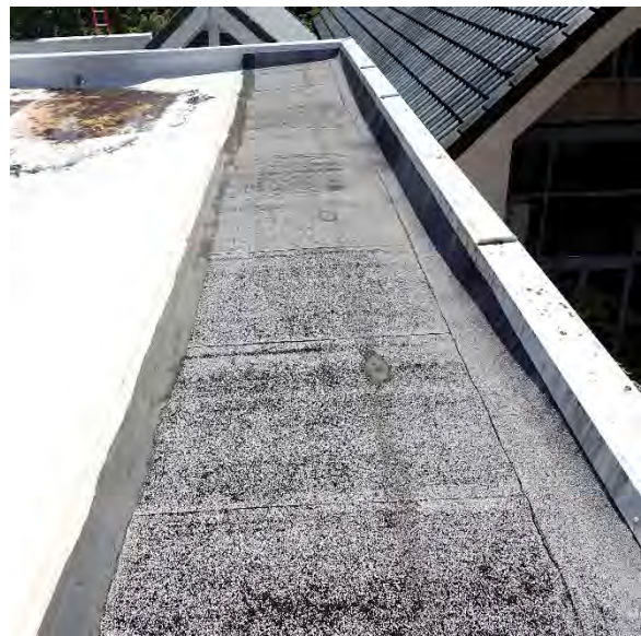
2.1B Additional view of decayed roof sheathing with previously patched holes.
