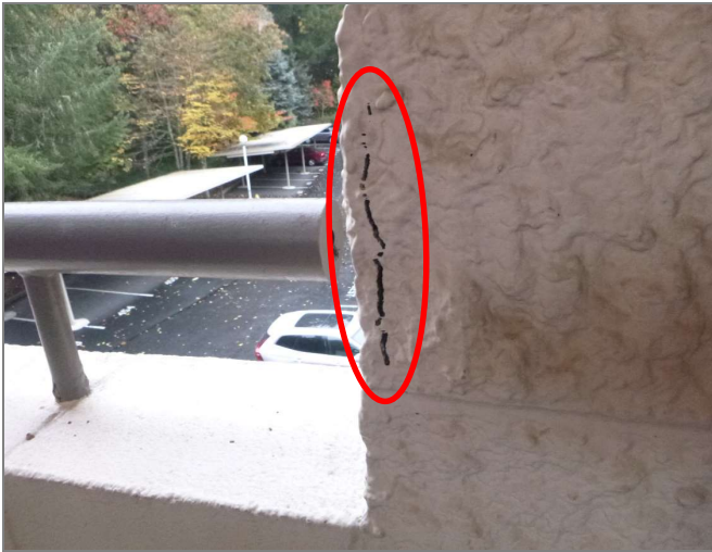
Figure 3.11 Building 5 Crack in coating and CMU at open-air corridor
