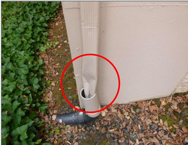
Figure 3.90 Building 5 Damaged downspout at transition to grade
