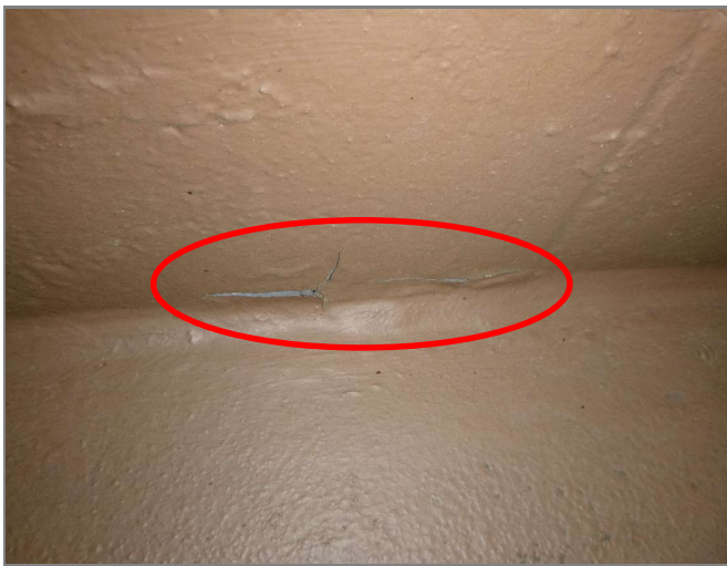
Figure 3.62 Unit 524 Failed coating at floor to wall transition
