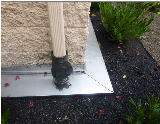
Figure 3.112 Building 1 Downspout penetrates base flashing
