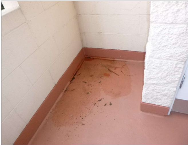
Figure 3.61 Unit 456 Standing water at balcony corner with no scupper
