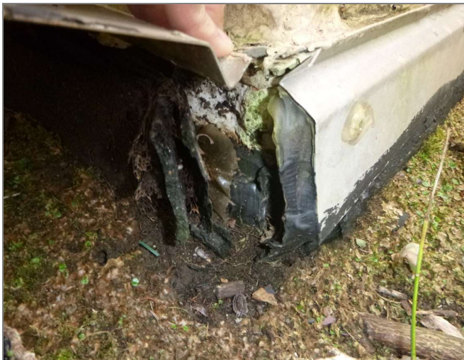
Figure 3.114 Building 4 Discontinuous termination bar with failed sealant
