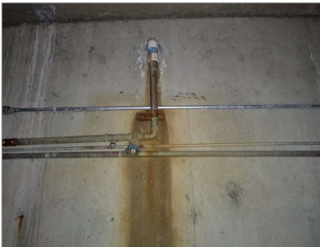
Figure 3.103 Building 4 Rust staining below conduit penetration at cast-in-place concrete wall
