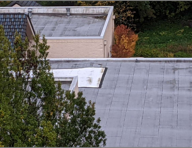
Figure 3.95 Apparent repair patch at center of roof area.
