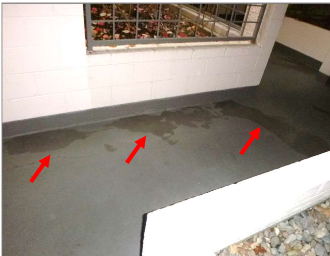
Figure 3.67 Building 5 Lack of slope resulting in poor drainage
