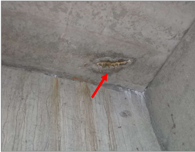
Figure 3.101 Building 3 Mineral deposits at underside of hollow-core slab
