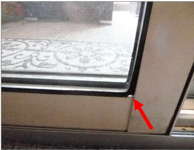
Figure 3.39 Unit 143 Displaced rubber gasket
