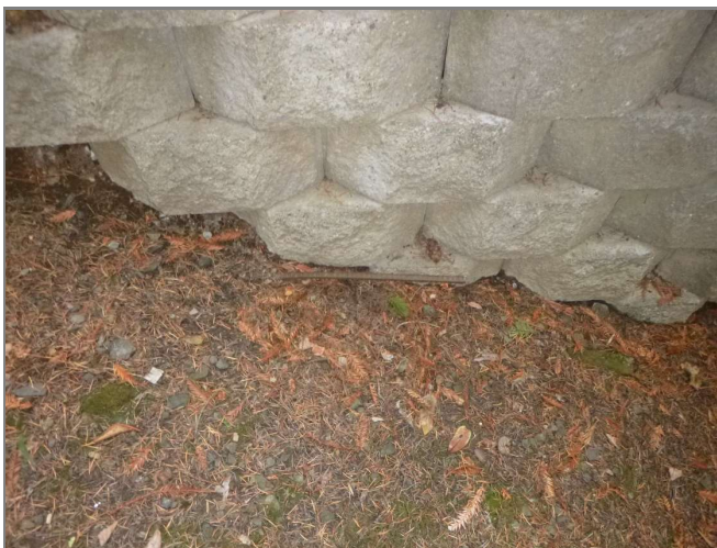
Figure 3.116 Building 4 Exposed rebar at retaining wall.
