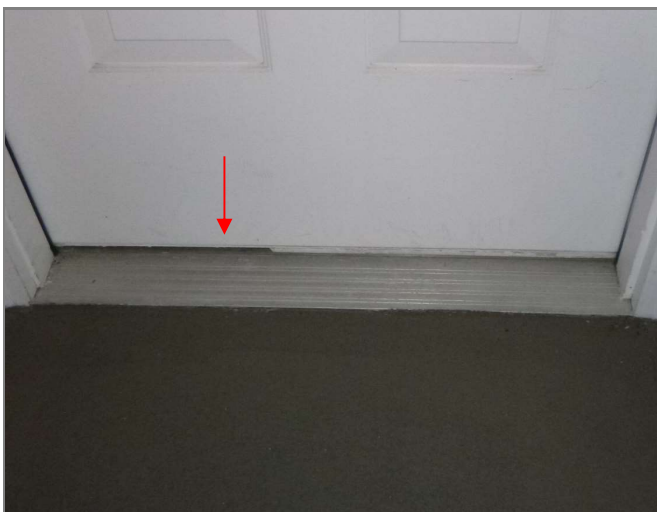
Figure 3.55 Unit 340 Damaged sweep
