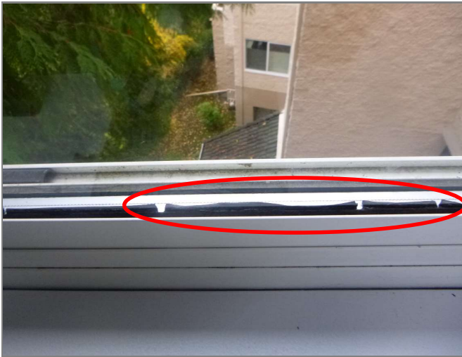
Figure 3.30 Unit 243 Failed glazing putty
