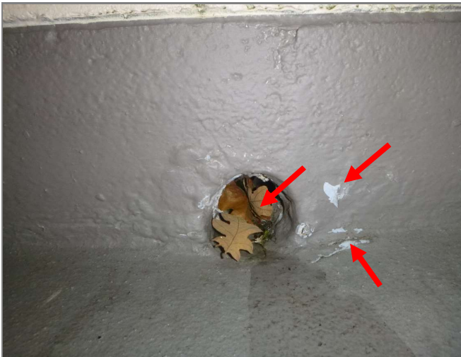
Figure 3.71 Building 5 Debris in scupper and failed coating at walkway
