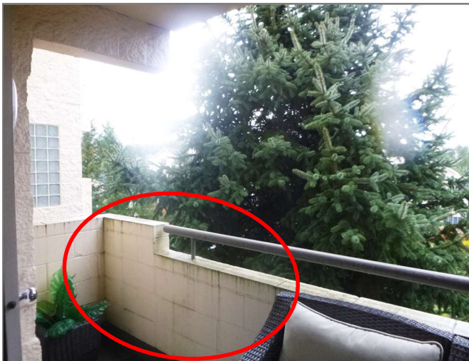
Figure 3.63 Unit 427 High levels of organic staining at balcony horizontal and vertical surfaces adjacent to tree
