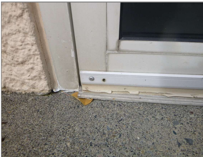
Figure 3.49 Clubhouse south elevation Failed sealants and sweep.
