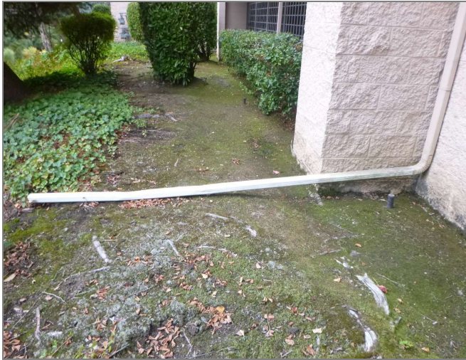
Figure 3.92 Building 4 Extension on downspout where grade slopes back towards building
