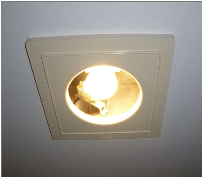
Figure 3.2 Typical original bathroom fan unit with bulb heater
