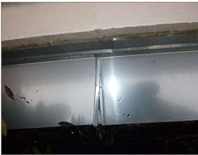
Figure 3.111 Building 1 Failed sealant and flat seam at base flashing lap
