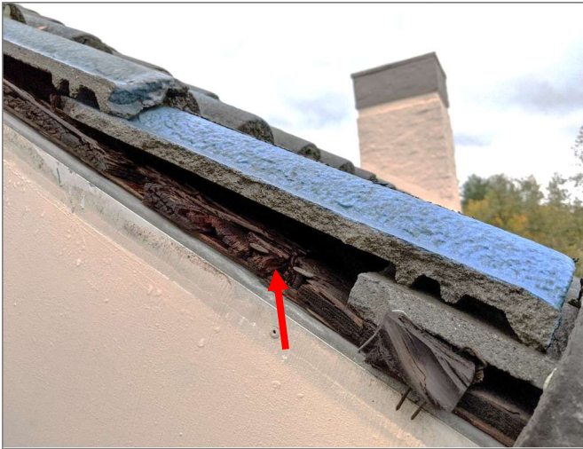
Figure 3.86 Building 2 Missing tiles at gable end reveal deteriorated plywood sheathing
