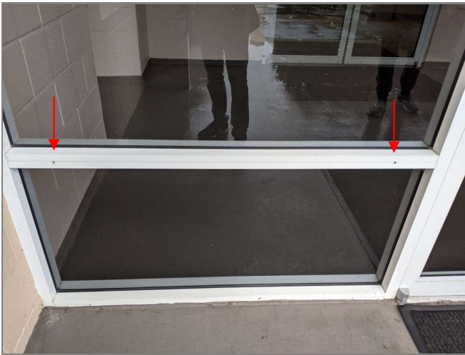
Figure 3.46 Building 1 Typical weeps.
