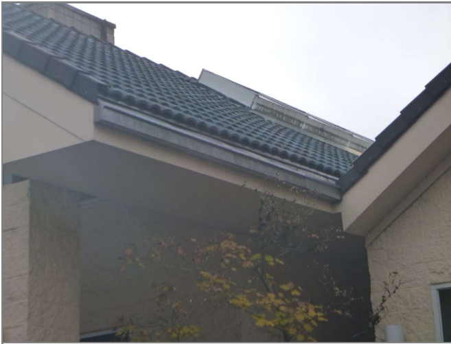
Figure 3.97 Clubhouse Gutter along main gabled roof at the entry does not appear to have any means to drain.
