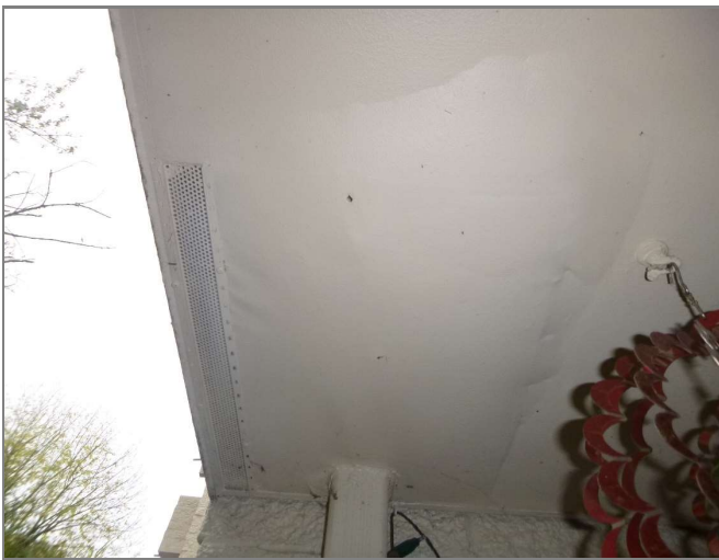
Figure 3.65 Unit 111 Large blister in coating at vented soffit with downspout penetration
