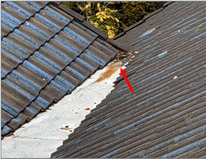
Figure 3.87 Debris and standing water at cricket valley between adjacent gabled roofs
