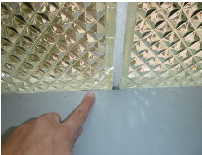
Figure 3.20 Unit 327 Minor cracks present at glass blocks
