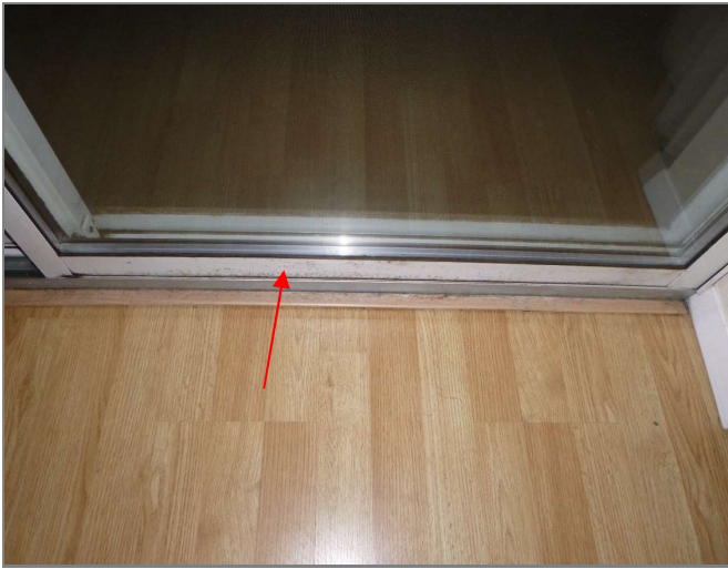
Figure 3.36 Unit 126 Organic growth/staining at frame.
