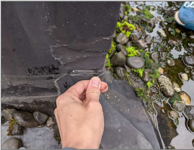
Figure 3.79 Building 2 Failed seal at roofing membrane corner up-turn detail
