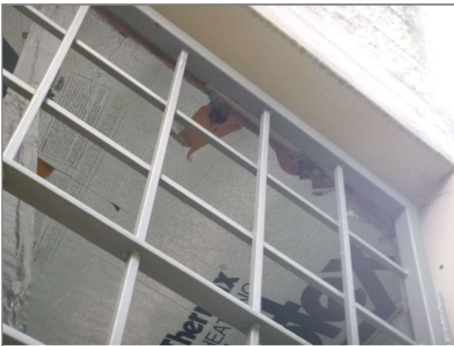
Figure 3.106 Building 4 Discontinuous and damaged insulation board at edge of parking garage.
