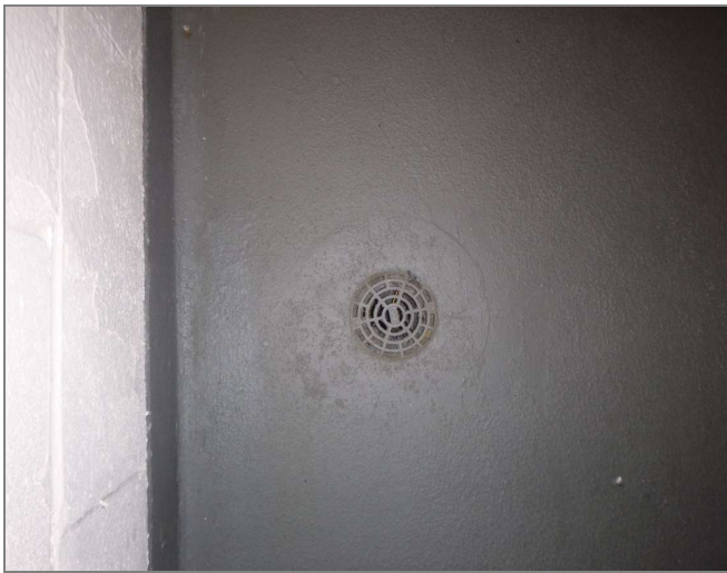
Figure 3.68 Building 5 Typical floor drain.
