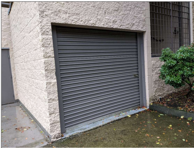
Figure 3.56 Building 1 Typical overhead coiling door.
