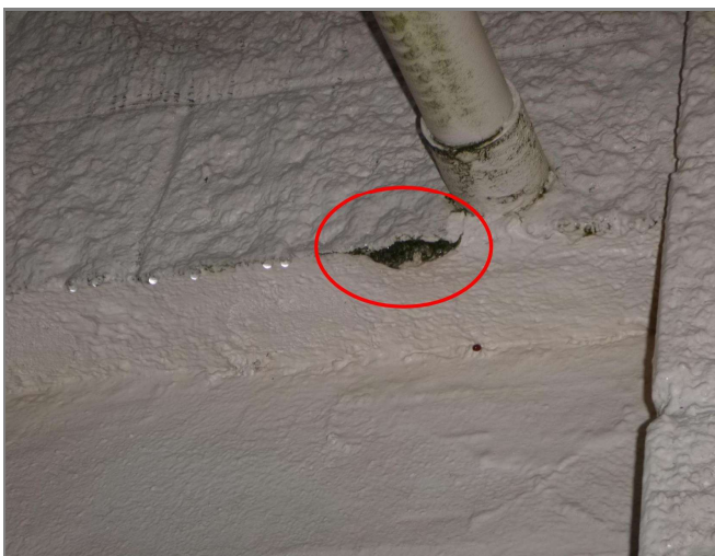
Figure 3.10 Building 1 Failed coating below scupper at open-air corridor
