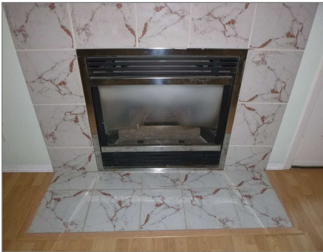
Figure 3.3 Unit 340 Fogging observed in gas fireplace
