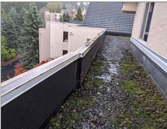
Figure 3.83 Building 3 Typical unwanted organic growth and standing water on roof ballast
