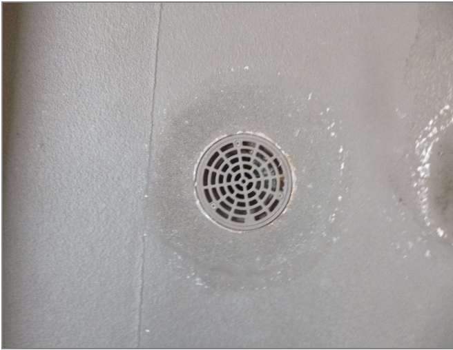
Figure 3.73 Building 1 Chipped and worn coating at drain flange.
