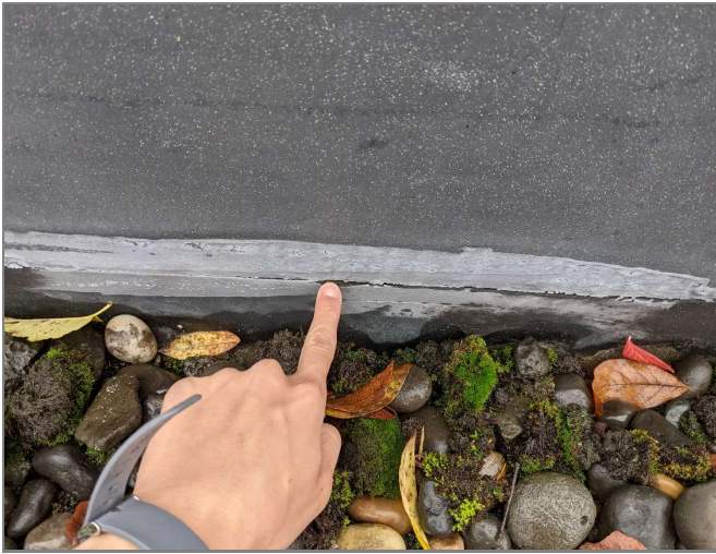
Figure 3.78 Building 2 Failed seal at patch to roofing membrane
