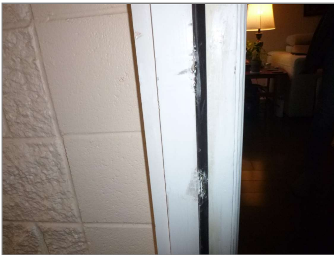
Figure 3.54 Unit 216 Damaged weatherstripping
