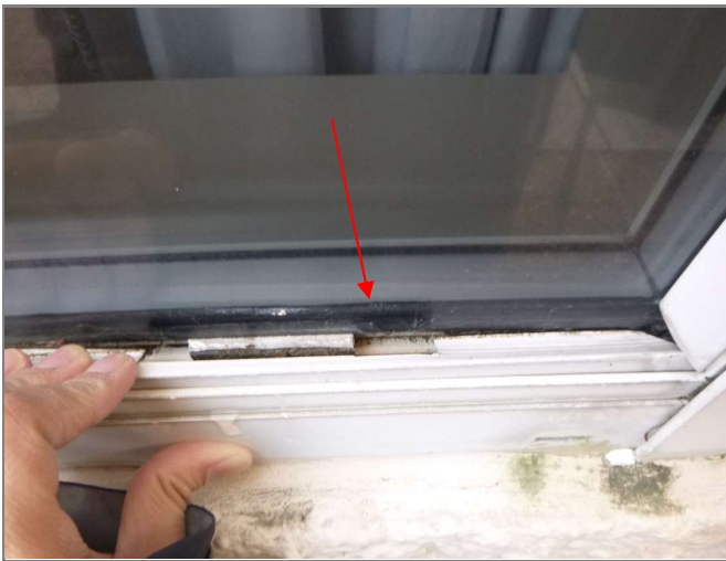
Figure 3.31 Clubhouse west elevation. Damaged glazing cap leading to missing/discontinuous glazing gasket.
