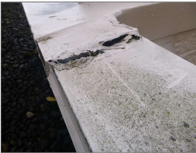
Figure 3.82 Building 2 Failed sealant at coping lap
