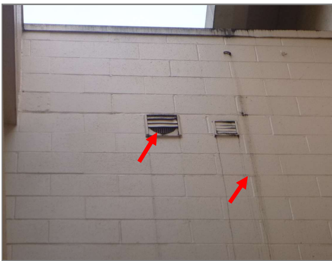
Figure 3.17 Building 1, Level 5 Missing slats and staining at exhaust vents in open-air corridor
