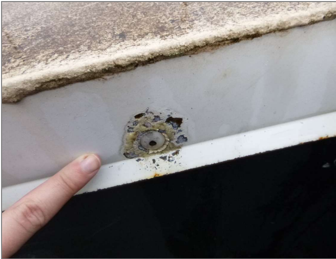
Figure 3.81 Building 4 Missing sealant at flashing fastener
