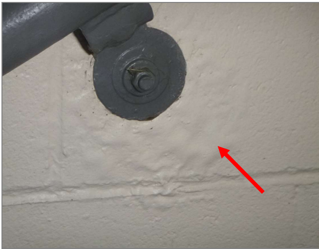
Figure 3.8 Building 1 Blistering coating at open-air corridor stairwell
