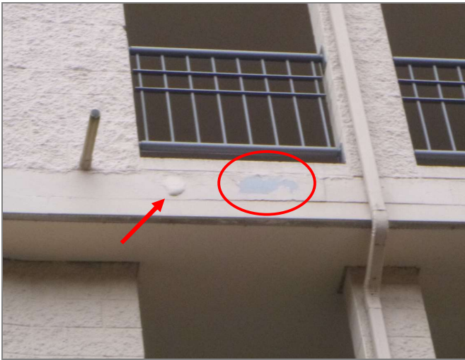
Figure 3.6 Building 3 Peeled and blistering coating
