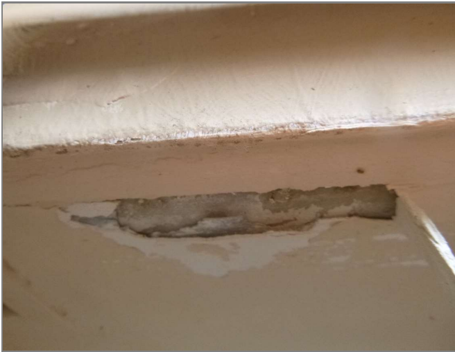
Figure 3.74 Building 1 Failed coating and spalling gypsum board at corridor ceiling
