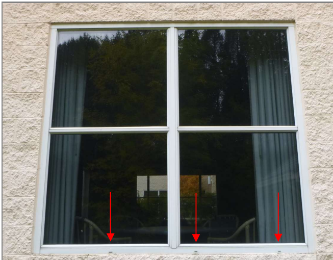
Figure 3.28 Clubhouse south elevation 4-pane exterior-glazed fixed windows. Note inconsistently spaced weeps.
