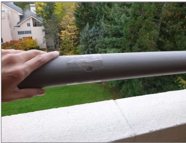
Figure 3.24 Unit 456 Worn handrail coating. Tape added by Owner.
