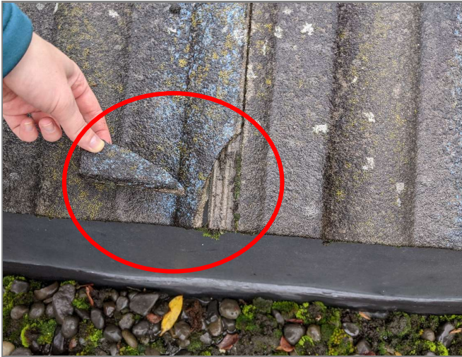
Figure 3.84 Cracked concrete tile at Building 2 roof
