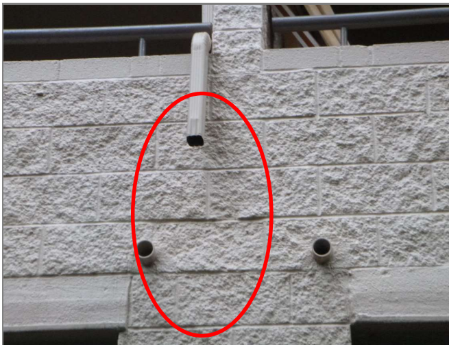
Figure 3.91 Building 2 Missing section of downspout
