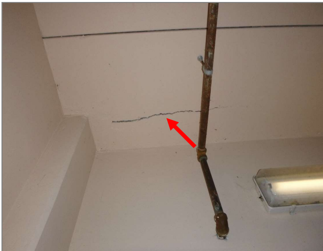
Figure 3.107 Building 3 Crack at stairwell
