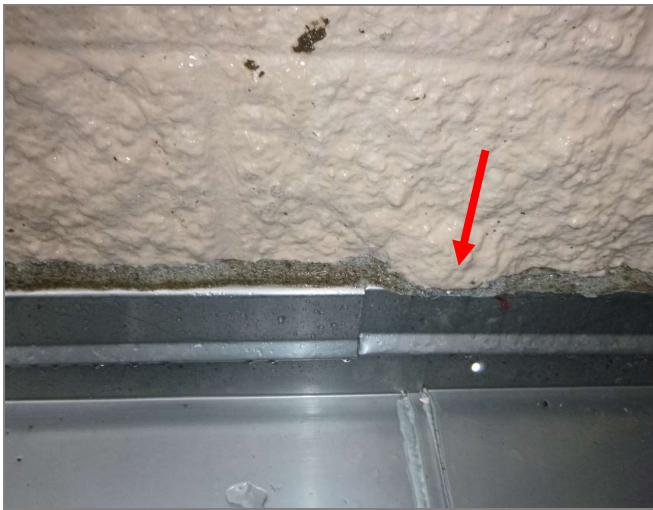
Figure 3.110 Building 1 Inconsistent sealant fillet bead width at new counterflashing.
