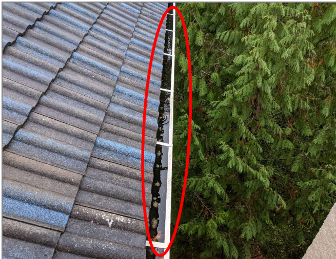
Figure 3.93 Building 2 Standing water in gutter at sloped roof
