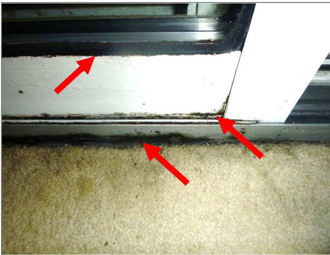
Figure 3.38 Unit 427 Condensation and organic growth on sliding door glass, sliding door frame, and carpet
