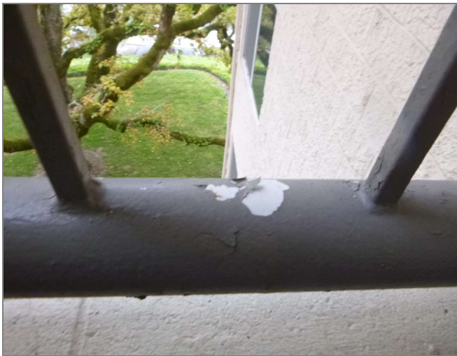
Figure 3.23 Building 5 Peeled coating at metal railing
