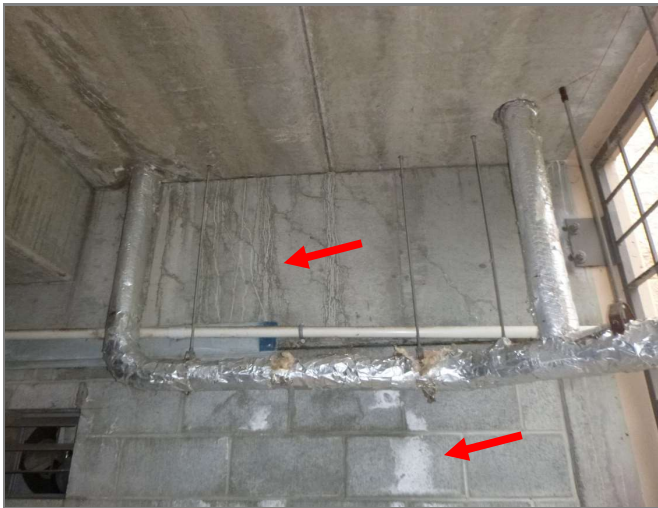
Figure 3.102 Building 3 Efflorescence and staining at the cast-in-place concrete and CMU walls
