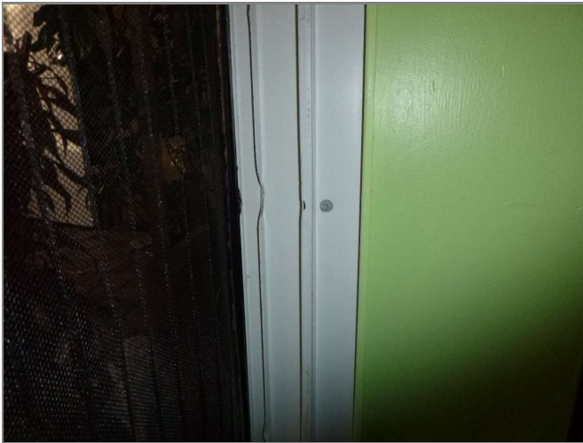
Figure 3.37 Unit 216 Damage to aluminum frame and door gasket.
