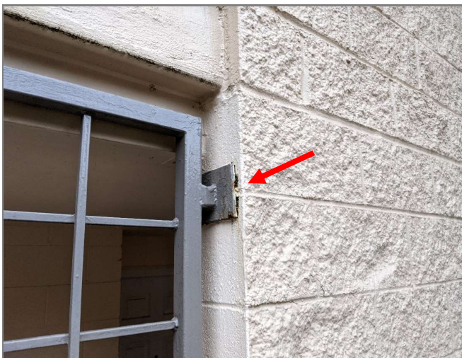
Figure 3.22 Building 1 Failed seal at corroding metal anchor mounts
