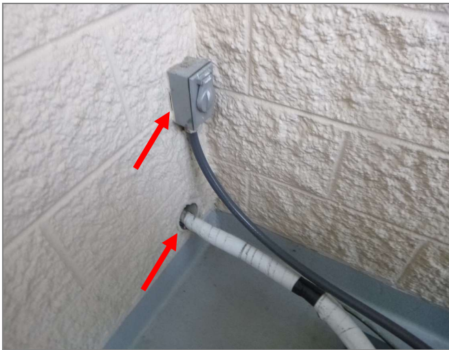
Figure 3.16 Building 4 Failed and missing sealant at conduit penetrations at balcony wall
