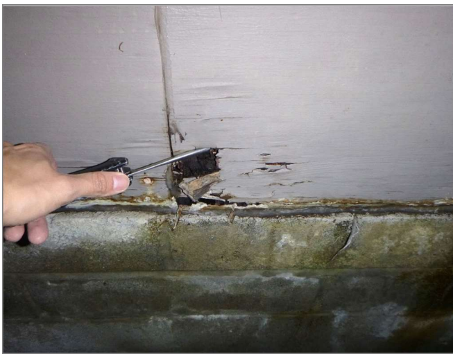
Figure 3.108 Building 5 Deteriorated plywood installed in wall opening
