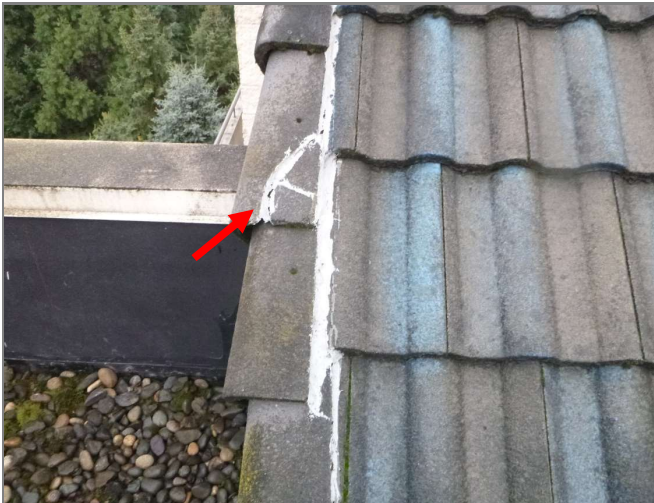
Figure 3.85 Building 5 Failed sealant repair at concrete tiles. Sealant is not a permanent solution to address leaks between concrete tiles.
