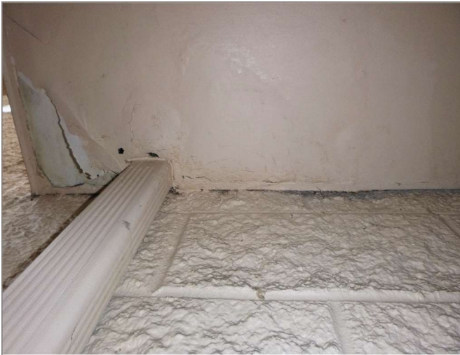
Figure 3.64 Unit 520 Blistering coating and gypsum board at soffit with downspout penetration
