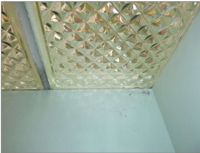
Figure 3.21 Unit 340 Localized black organic growth at mortar and windows, indicating ongoing condensation issues.
