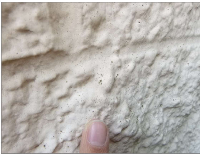
Figure 3.9 Clubhouse UV degradation resulting in pinholes in coating.
