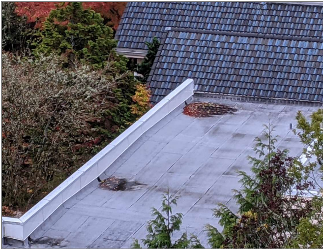
Figure 3.96 Debris accumulation at scuppers.
