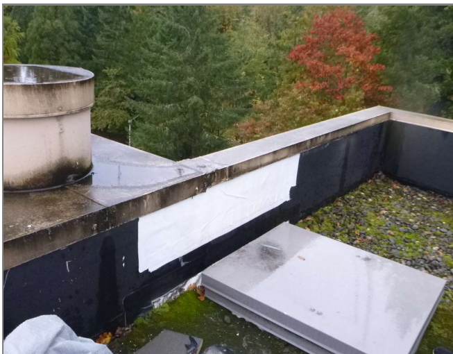
Figure 3.77 Building 5 Temporary patch of self-adhesive material.
