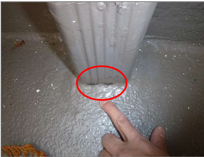
Figure 3.59 Unit 340 Failed coating at downspout penetration
