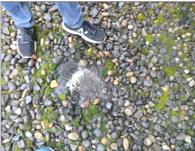
Figure 3.80 Building 5 Crack repair in EPDM membrane. UV degradation (crazing) is present due to exposure.
