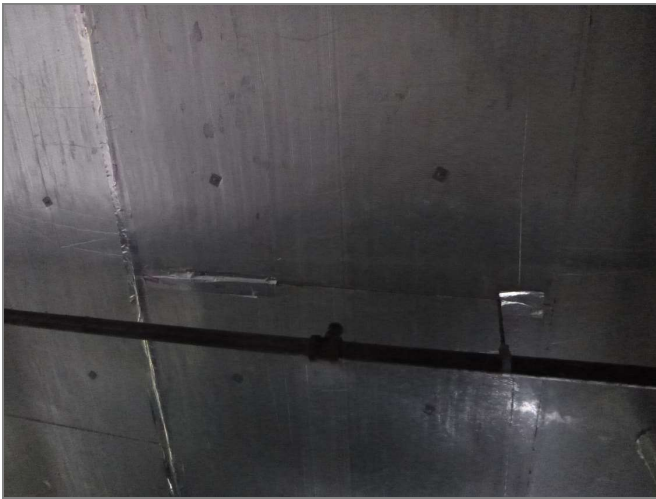
Figure 3.105 Building 1 Foil-faced insulation boards applied to underside of conditioned space. Foil tape is discontinuous.
