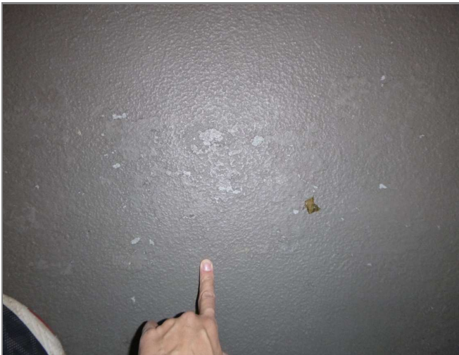
Figure 3.72 Typical localized failure of coating at open-air corridor floors where coating is worn off, revealing the lighter surface below
