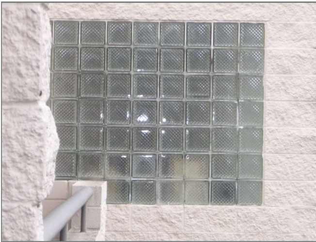
Figure 3.19 Adjacent to Unit 456 Fogging present in glass blocks.
