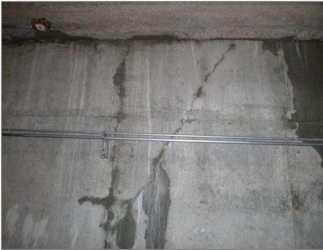
Figure 3.104 Building 1 Water leaking through crack at cast-in-place concrete wall
