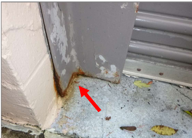
Figure 3.57 Building 1 Corrosion at coiling door frame.
