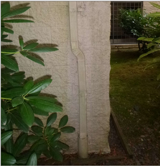
Figure 3.12 Building 5 Organic staining at exterior CMU wall
